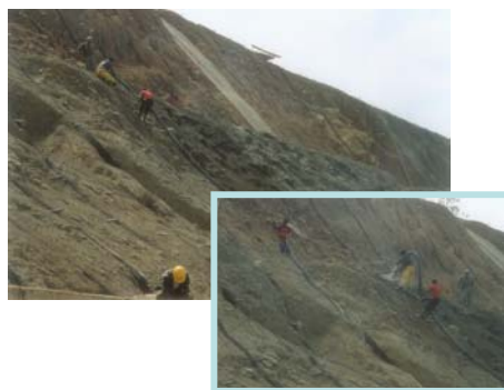
Fig.9 Use of anchored mesh and gunite to reduce infiltration of water and maintain stability on the back-slopes of the highway in Ecuador. Placing gunite on the back-slope consisting of residual soil
