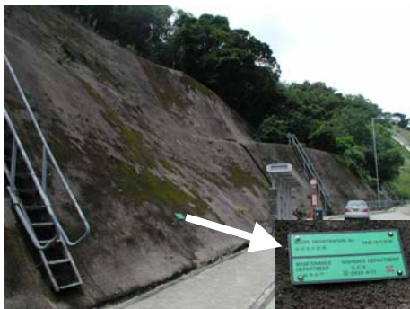
Fig.20 Identification plaques placed on the surface of a slope to assist the public in participation in slope management. Each slope is photographed from a variety of angles and has an identifying label. Performance data is stored in a large database
