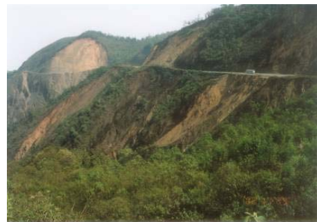
Fig.6 Another example of almost continuous slope instability triggered by changing geometric and environmental conditions along the highway in Ecuador
